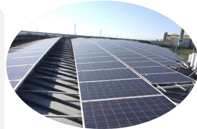
Taichung Wujih Solar Photovoltaic Plant
