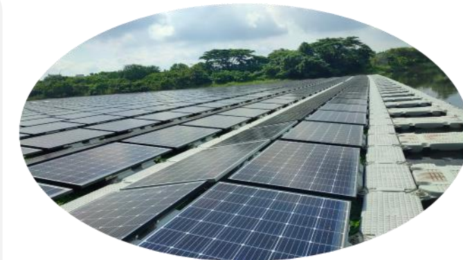
Tainan Tree Valley Park Solar Photovoltaic Plant
